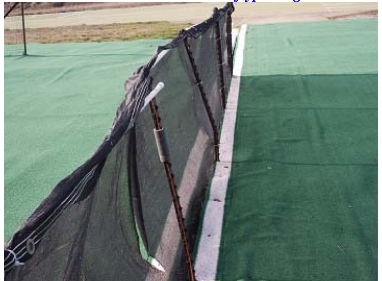
A storm went by and the wind bent the wind break fence between the hot and cold pit areas.
