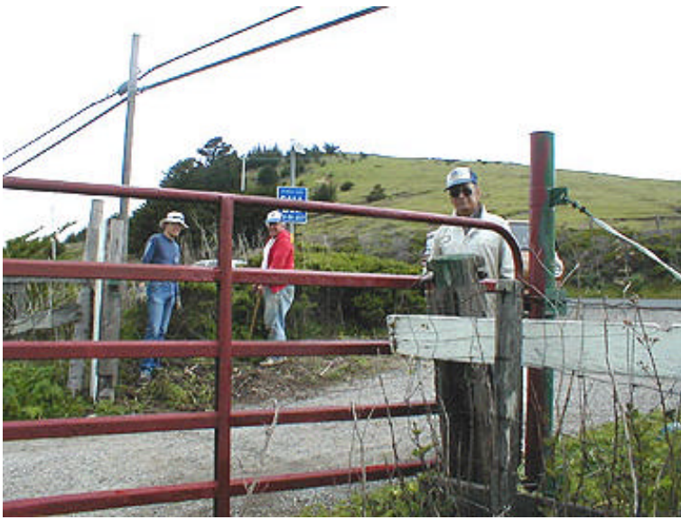
Ken, Eric and Lou repainted the gate and removed the vegetation around the driveway area. Looking good!!!
