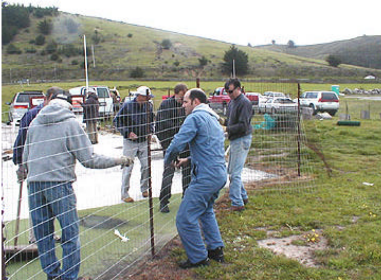
The guys installing new wire mesh to protect us from those bad landings from the south.
